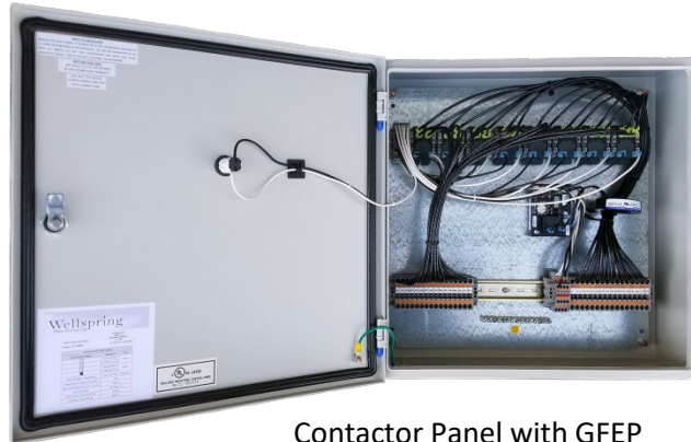
Contactor Panel with GFP
